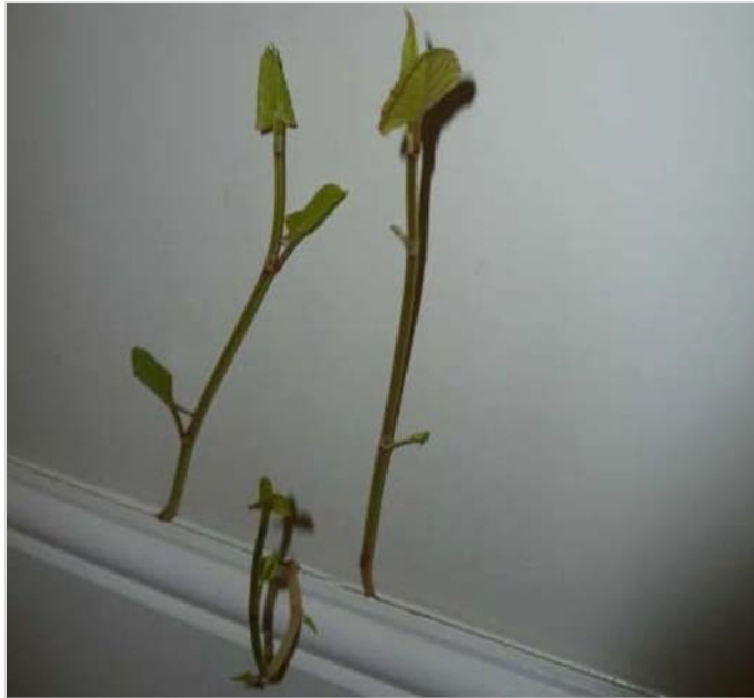
2a. House wall breached by Japanese Knotweed.
