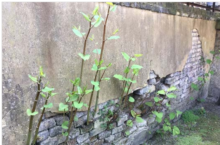
2c. Retaining wall pierced by Japanese Knotweed.
