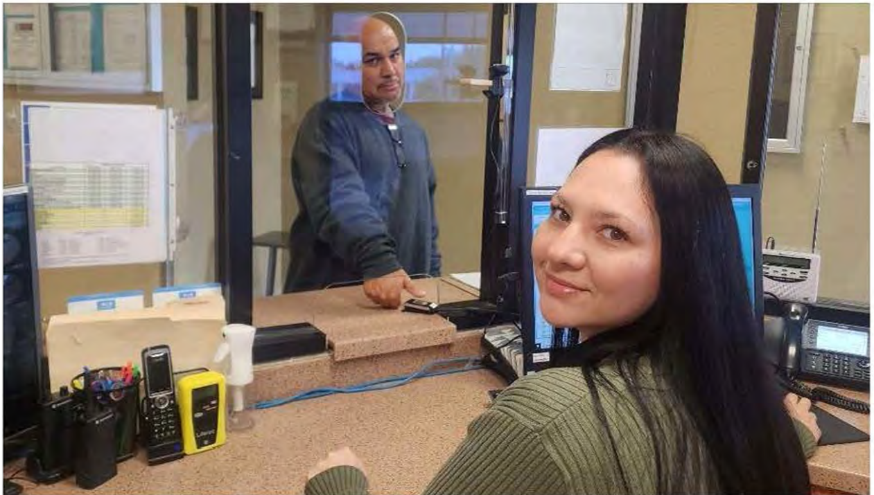
Typical Secure Central Monitoring Office (CMO) showing Transaction and Observation Windows to Main Entrance, Reception Area, Security Camera Monitor, multi-line Staff Telephone system with Intercom/Paging capability, Alco Blow Evidential Breath Measurement Device and a Hand-Held Metal Detector. The CMO monitors all client, team member, vendor and visitor movement in and out of the RRC. A Resident Monitor is shown checking a client out of the RRC using the Resident Accountability Module (RAM) fingerprint scanner to identify the client and confirm their approved movement schedule.
