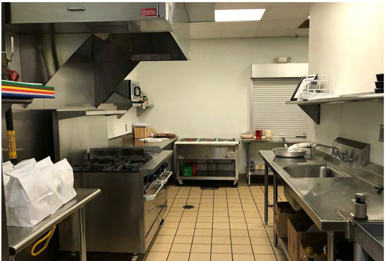
Typical Full Service, Commercial Kitchen is equipped with High Quality, Stainless Steel Equipment
