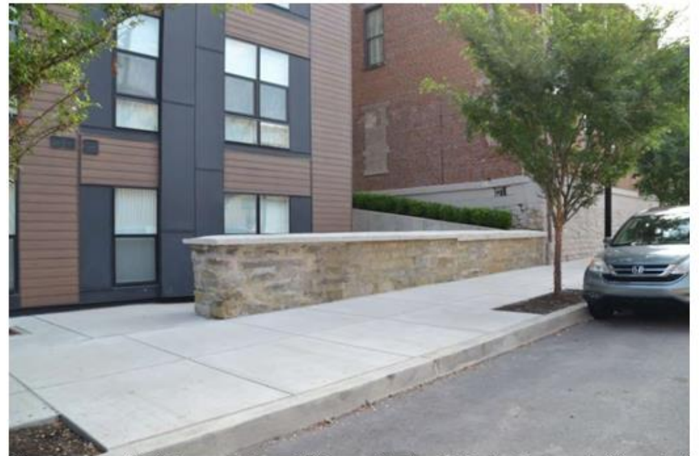
Photo 3: Stone Wall Segment along 39 th Street, North of Officer's Quarters Building, Looking Southeast
